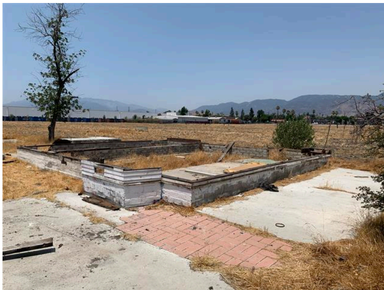
Photo #8 View of concrete residential building foundations located in southeastern portion of the Property. View looking to the northwest.
